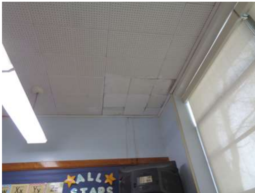
Photograph 2: Ceiling Tiles in Room 17.
