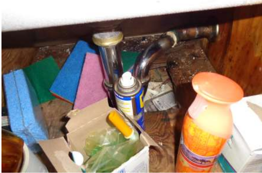
Photograph 5: Wood shelving below classroom sink in Room 9.
