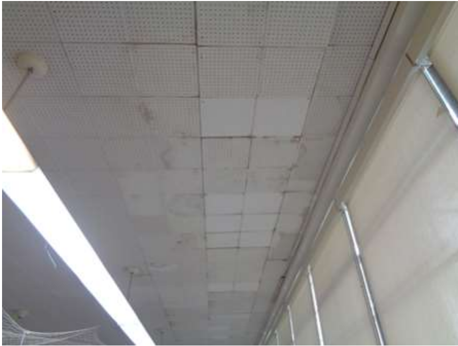
Photograph 1: Ceiling Tiles in Room 10.
