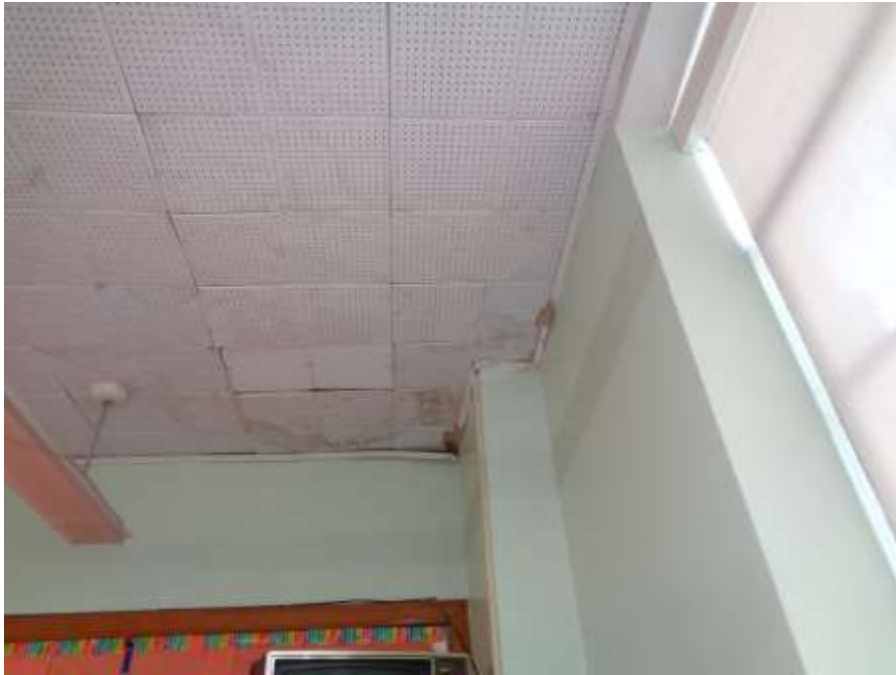
Photograph 3: Ceiling Tiles in Room 9.
